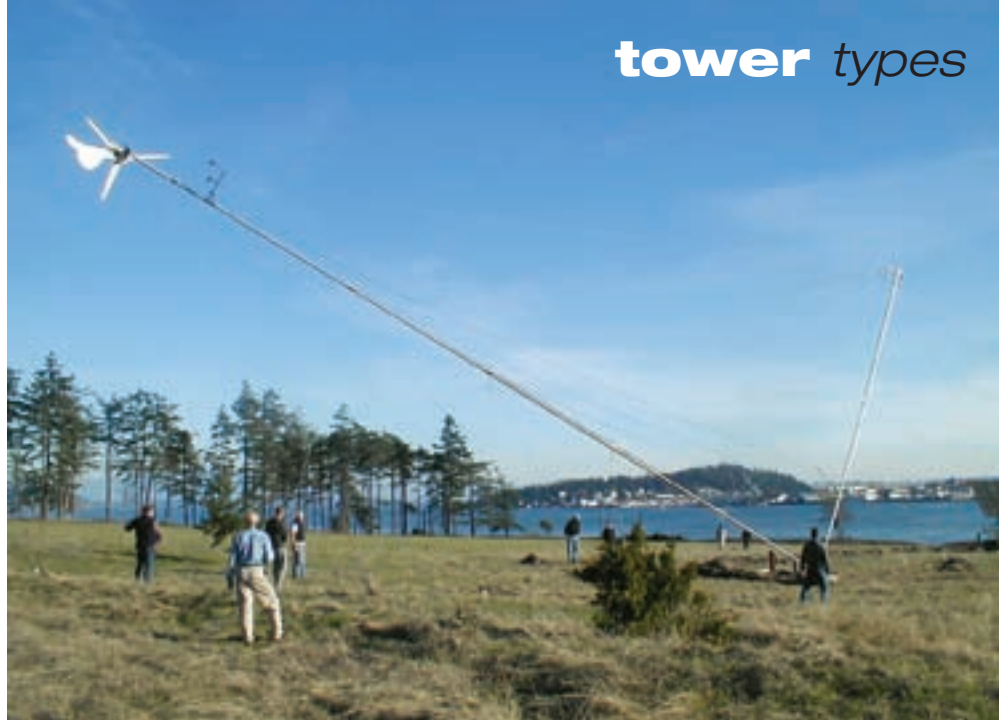
As the gin pole goes down, the tower goes up—tilt-up towers need wide open and level spaces, but make installation and maintenance easy.
